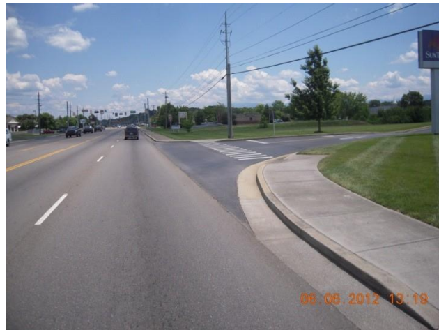
This driveway does not maintain the curb and gutter through the entrance.
